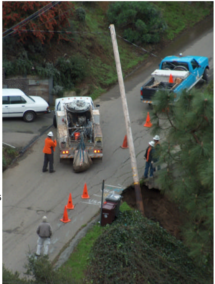
PG&E crews work to stabilize the leaning power pole. Photo by Eric Choate
